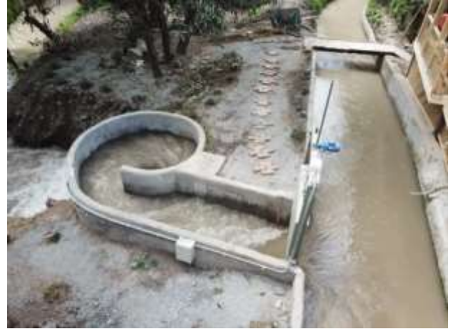
Fig. 5- Picture of a vortex turbine generator [13]
