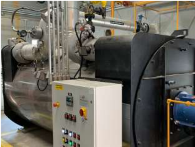
Fig 3. Thermal fluids heaters [9]
