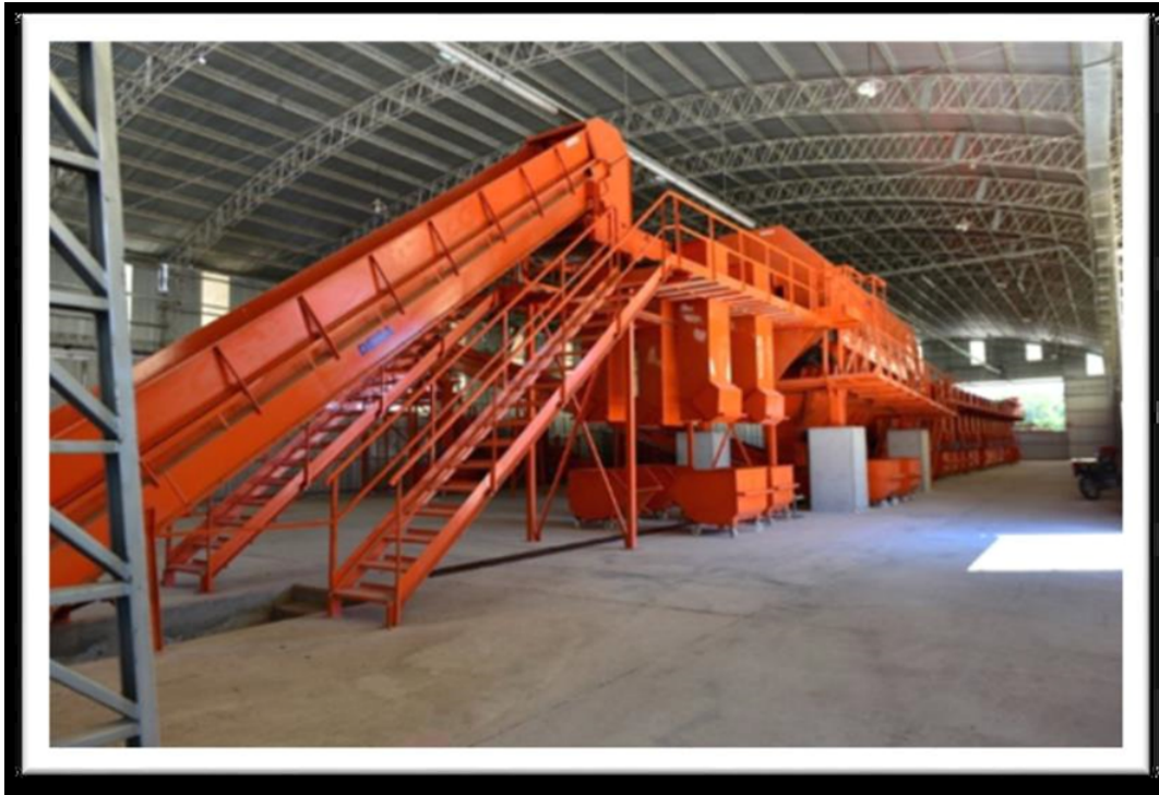
Fig. 19. Machinery used in the plant [1]
