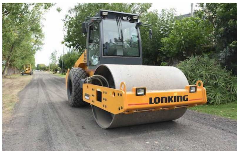
Figure 1. RAP use only, distributed with a motor grader and compacted with a smooth roller in a suburban area in the Municipality of Berisso (Buenos Aires, Argentina)
