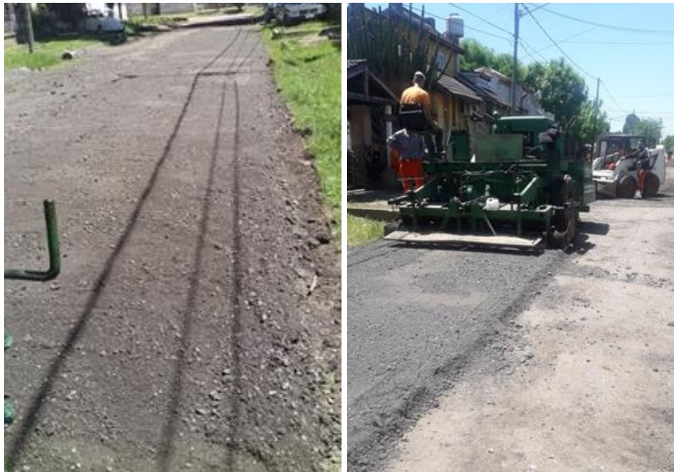
Figure 3. RAP use plus used car oil, distributed with a finisher in a suburban area in Gran Buenos Aires (Argentina)
