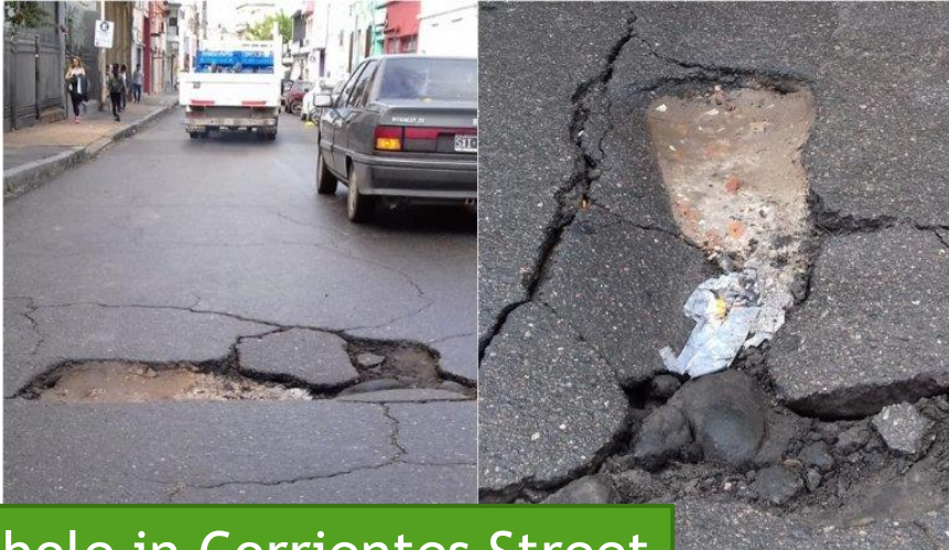
Pothole in Corrientes Street
