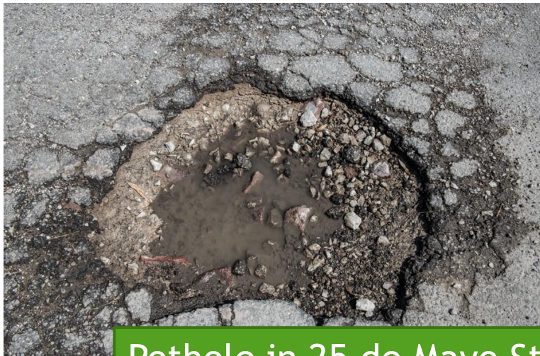
Pothole in 25 de Mayo Street
